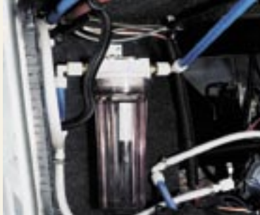
The water filtration system provides safe clean drinking water through all the water lines and water heater.
